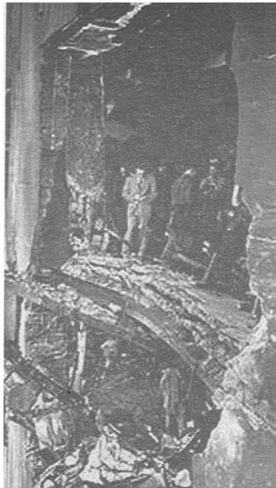
One of the R-25 engines, and part of the landing gear, went through the building, tearing a hole 18 by 20 feet
